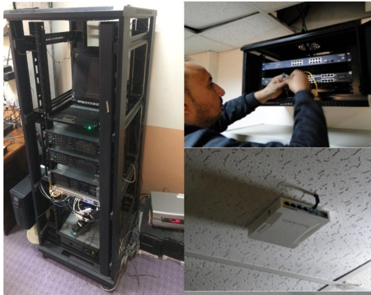
Fig. 2. Fiber optic and Wi-Fi installation.
